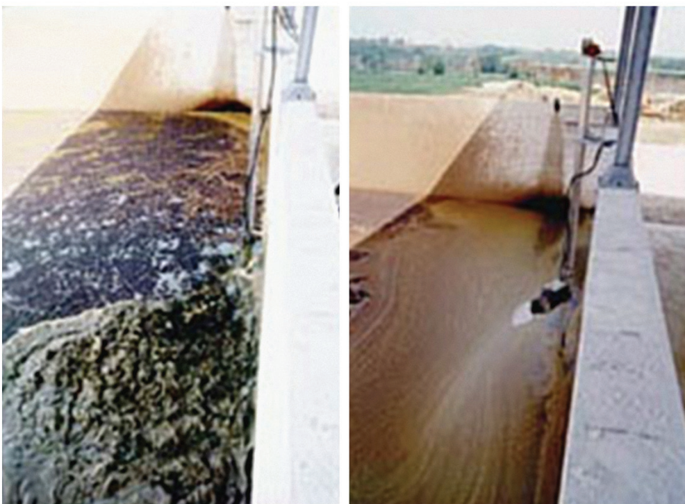
Before and after photos of TBM mixer installed in waste water pit.
